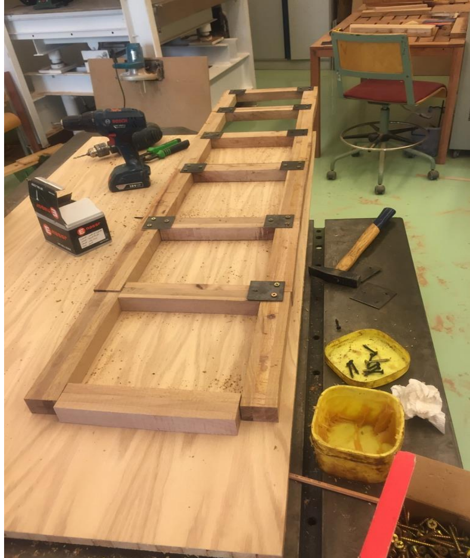
Figure 70: Building the external members of the truss and connecting them Then the inner diagonals are inserted and connected as shown in figure (71).
